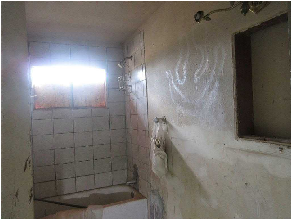
Photo 3: Interior view of a bathroom in the on-site dwelling. Evidence of previous water intrusion and visible minor mold growth is present.
