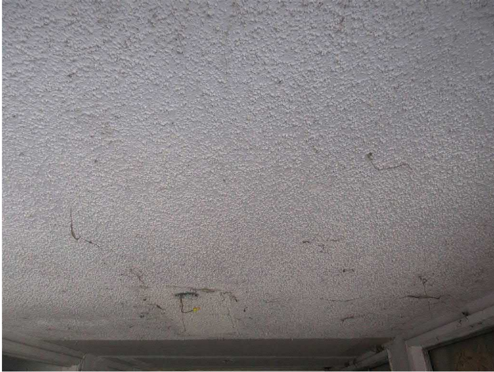
Photo 5: Interior view of a ceiling within the on-site dwelling on which blown (spray-on) ceiling material is present.
