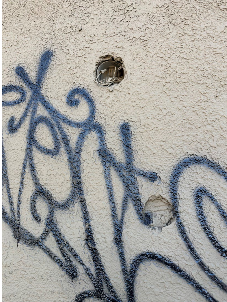
Pictured Above: Electrical wire vandalism and damages to the building example.
