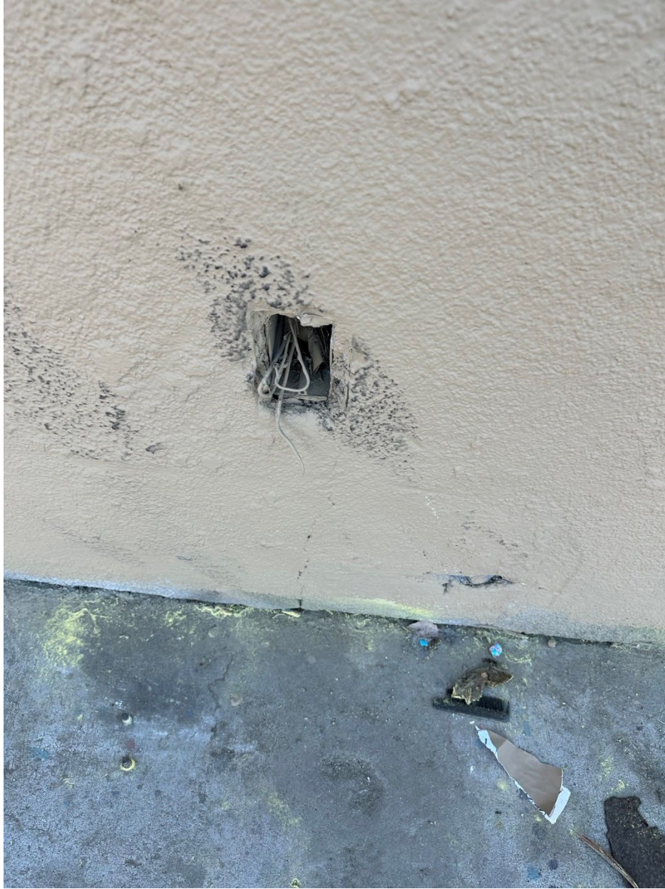
Pictured Above: Additional electrical wire vandalism and damages to the building example.
