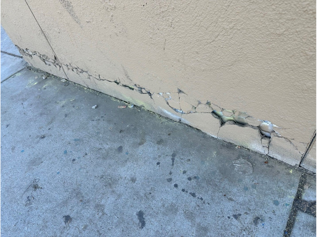
Pictured Above: Structural damage to the building example.
