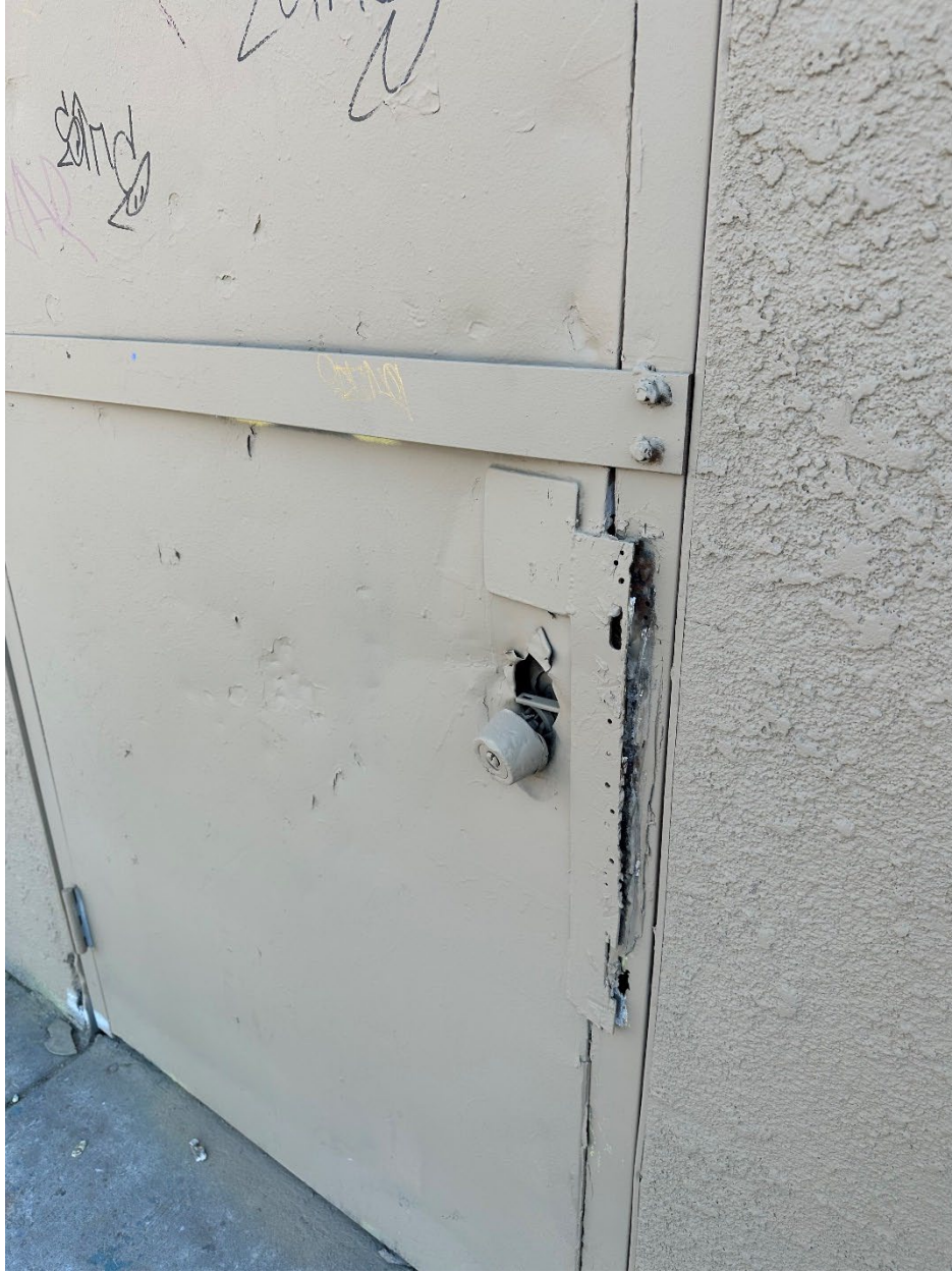
Pictures Above: Entrance door to the building has been welded shut for several years now to deter unauthorized entrances or vandalism to the inside of the building.
