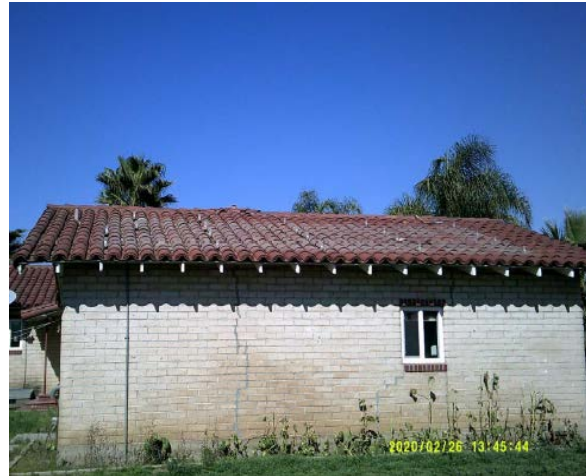
Picture 2. Panels Missing from Roof
