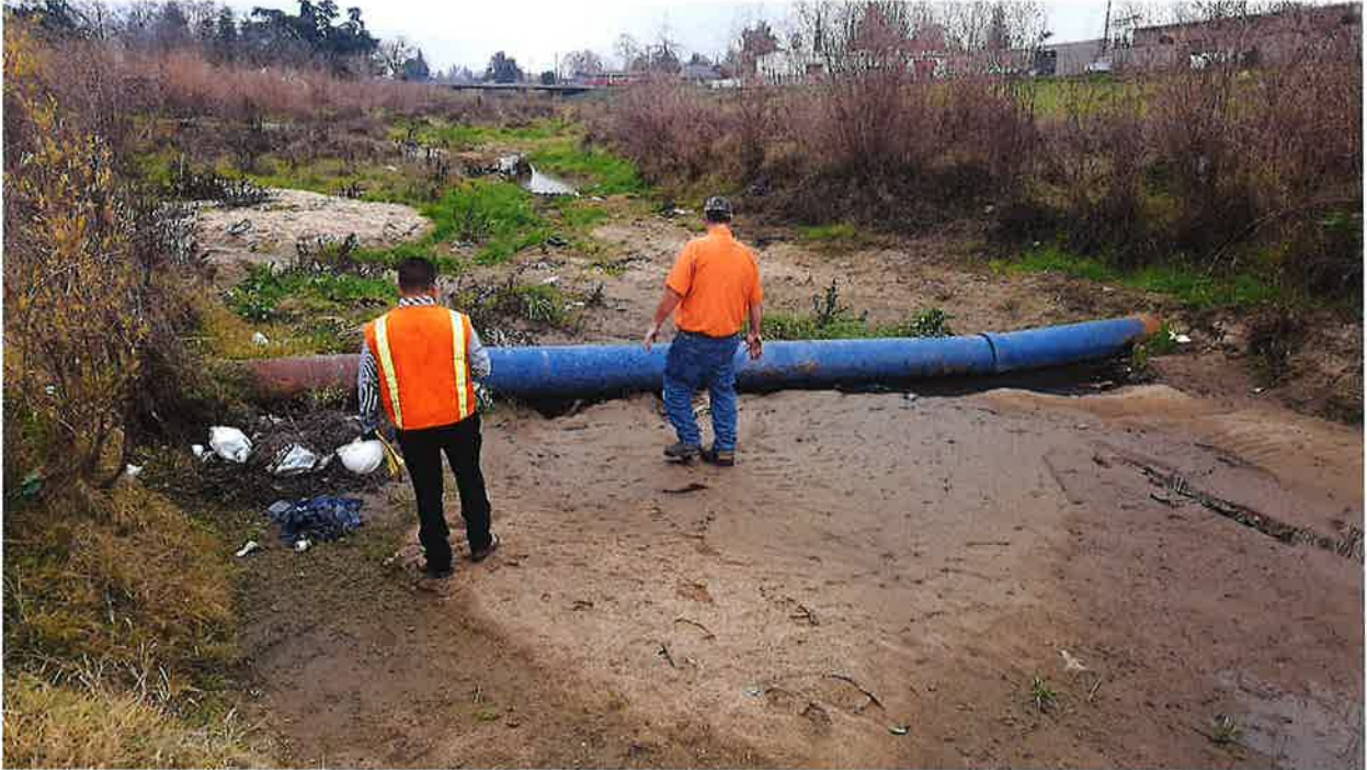
Figure 1 – Exposed 16-Inch Water Main at the Fresno River Channel
