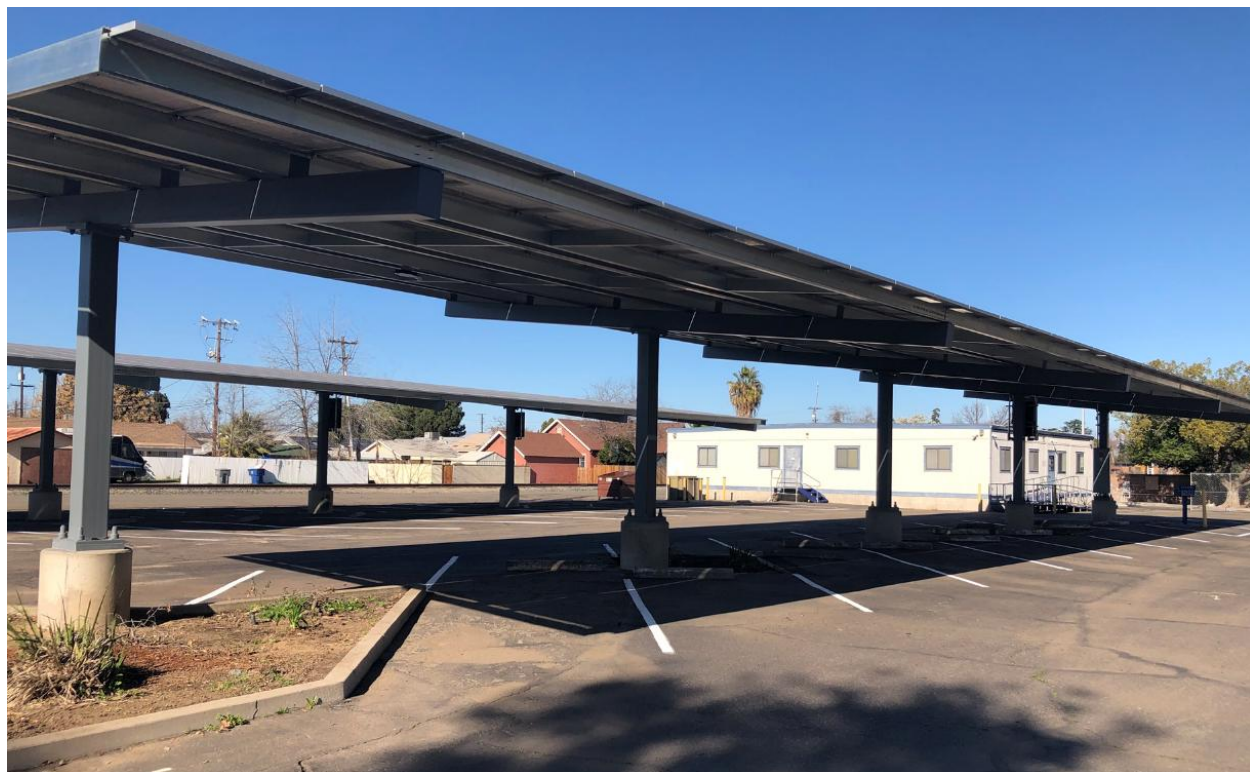
City Hall Solar Canopy
