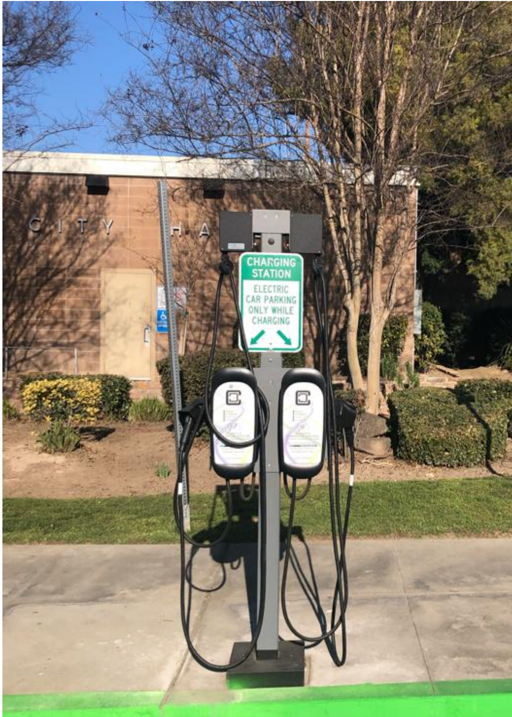
EV Charger City Hall
