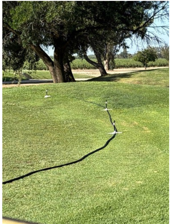
Strings of micro-sprinklers are being utilized around the putting greens to provide supplemental water to the surrounding turf.
